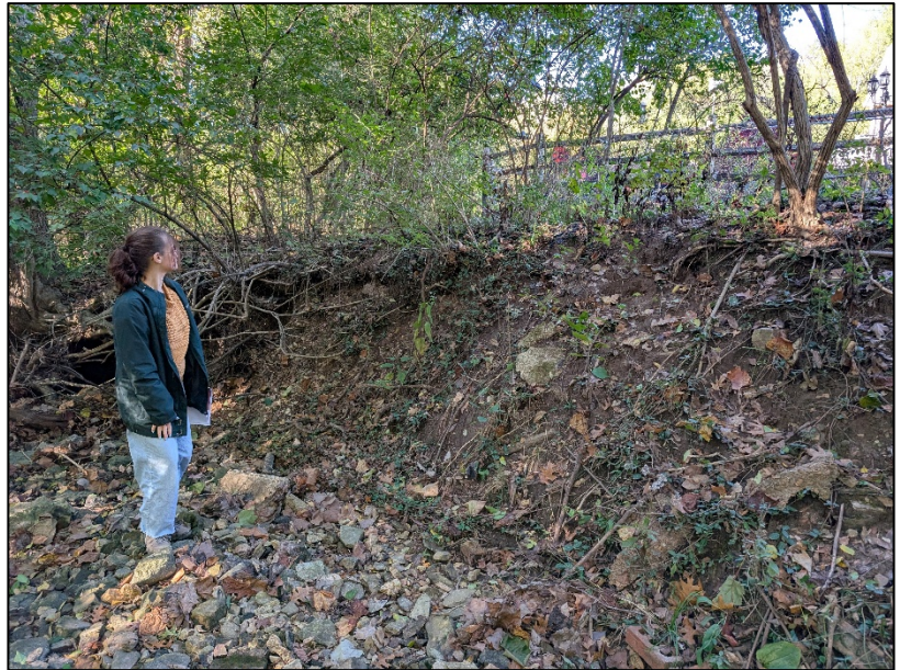
Photo 2: HR Green Engineer Observing Creek Erosion in Sunset Hills
